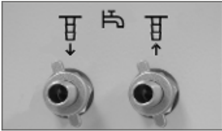
Fig. 66: Counter nuts on the cooling water nozzles
